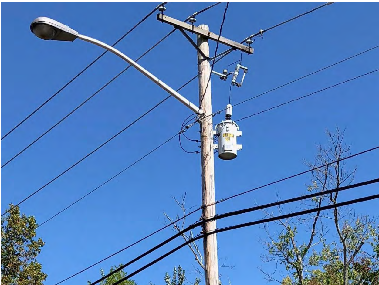
Figure 4.1 Typical NU Pole with Multiple Users Attached
